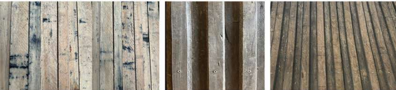
Example of metal staining to expect
